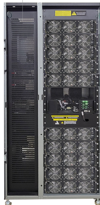
MEPSM10700 700kW UPS (door removed)
