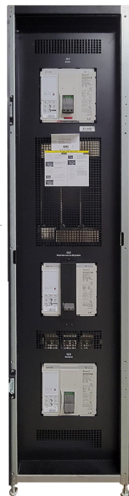
Maintenance bypass (door removed)
